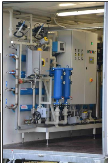
Fig. 3: View of equipment mobile membrane unit
